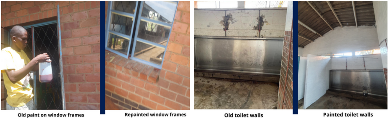
Old paint on window frames
