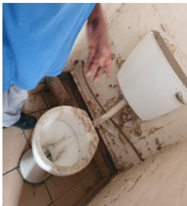
Old toilet seat
